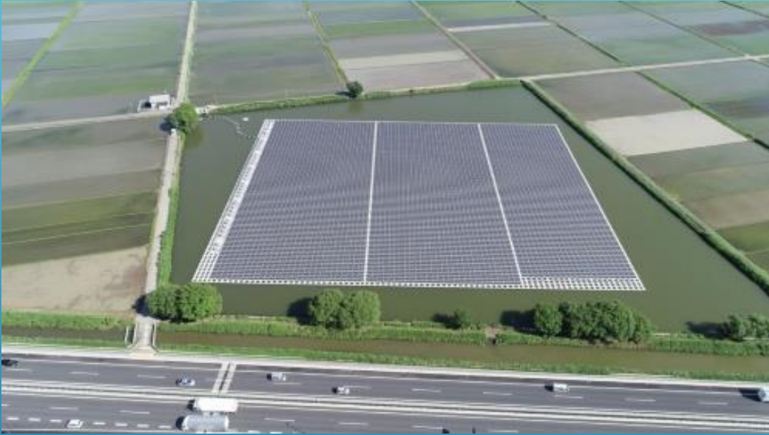
Kayamanuma Solar Power Plant (2.6MW) in Kuki City, Saitama Prefecture.
